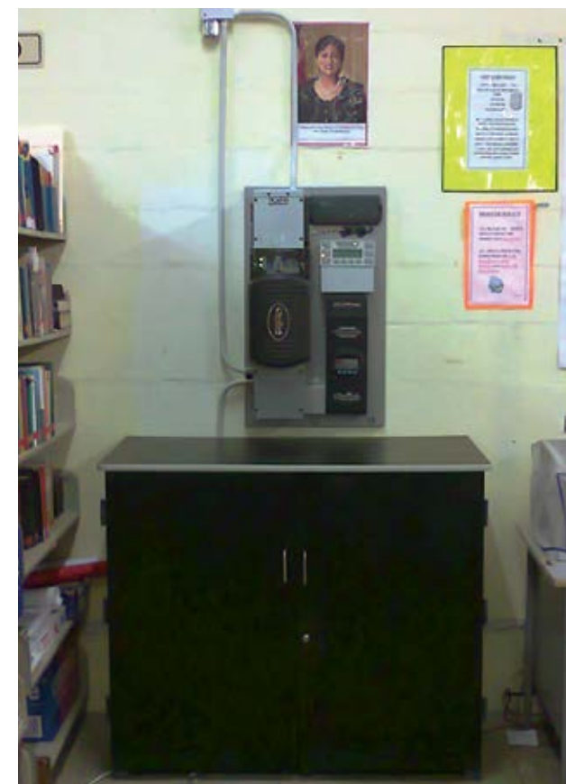
PV installation at North Eastern College.
